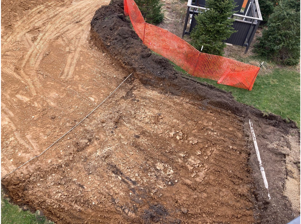
Electrical line and 4" water line impacted by the construction of the new playground.
